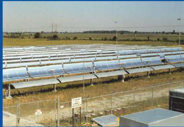
When the College was constructed, The Total Energy Solar Photovoltaic Conversion System was originally intended to power the College by generating both electricity and hot water. A total of 270 single-axis tracking concentrating collectors were installed, each measuring 20'x7'.
